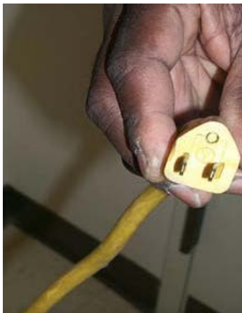
Fig. 1 Ground prong broken off
