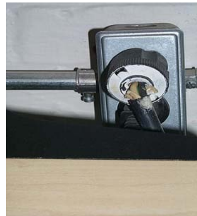
Fig. 2 Wire cover pulled from plug
