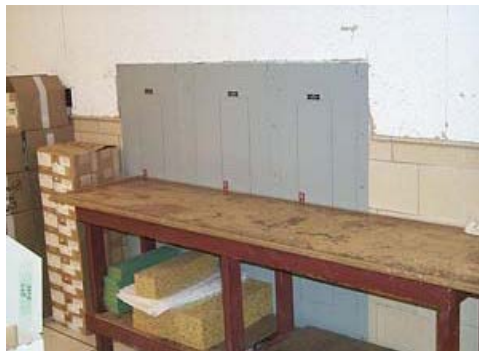
Figure 1: Blocked Electrical Panel
