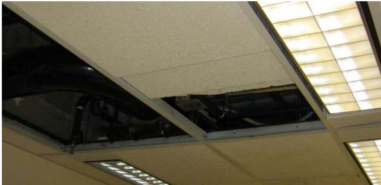
Missing and damaged ceiling tiles
